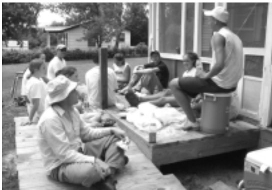
Lunch break on the work site included a devotional led by one of the teens.
