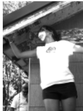
There was lots of old peeling paint to scrape off the houses.
