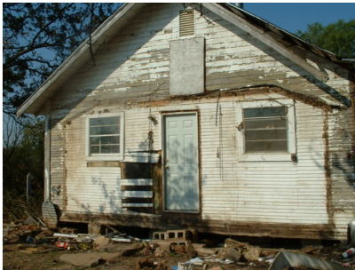
The dilapidated home needed a complete rehabilitation.
