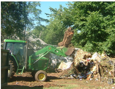
Tons of trash were removed before work could even begin on the house.
