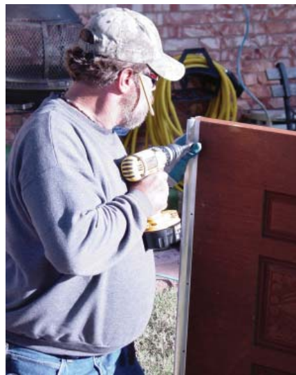
Gary Wirtz adds a door bottom to the front door of the home that will help seal out the cold weather.
