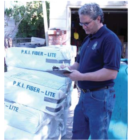
Matt Van Horn, Weatherization Coordinator for the Community Action Agency of Oklahoma City and Oklahoma/Canadian Counties, checks the supply of insulation to be added in the attic.
