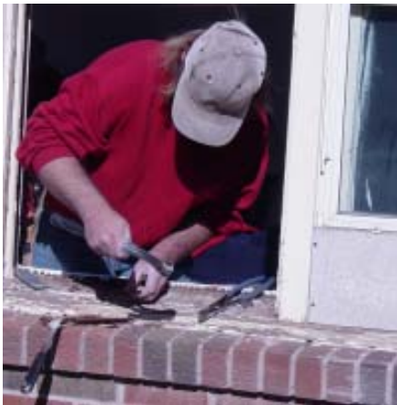
A Community Action Agency of Oklahoma City and Oklahoma/Canadian Counties weatherization crew member prepares to replace a broken window.
